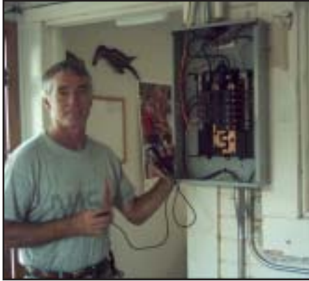
Bill Swanson shows off the new electrical panel he installed at Orchard House. Photo by Alice Elshoff.
